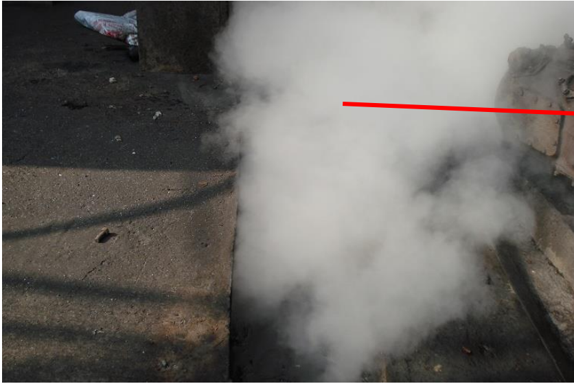
Before Installation Photos showing Steam Loss
